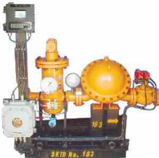
MSA meter skid with Toptech SMP controller
